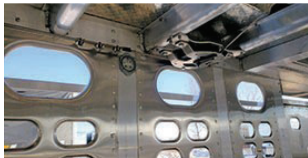
Single sheave assembly (mounted under stationary deck).
